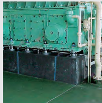
Gas engine on concrete
